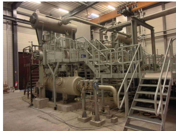
Figure 3: Compressor K-24 in the machine hall.
